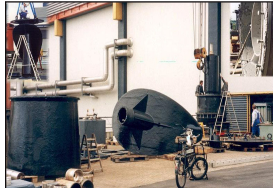
Completed application of ARC 858 and ARC 855 to all the wet end pump components
